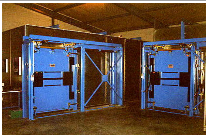
RF sliding doors on two EMC test chambers
