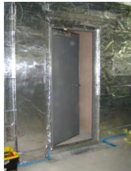
RF shielded door
