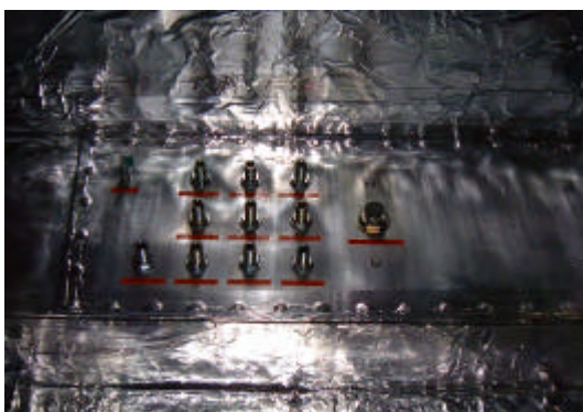
Penetration plate for FO cables and telephone filters
