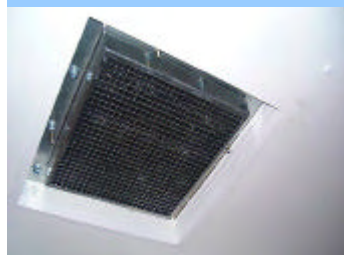
RF shielded ventilation vent
