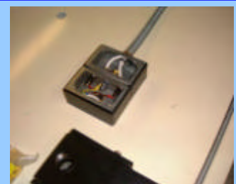
RF filter box for solenoid lock, designed to ensure no RF leakage on the wires through the door
