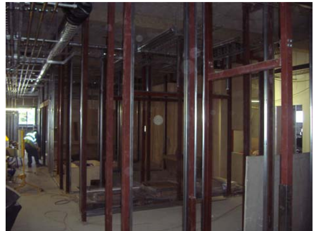
Steel framework for a PET scanner suite. Lead lined doors installed by EEP
