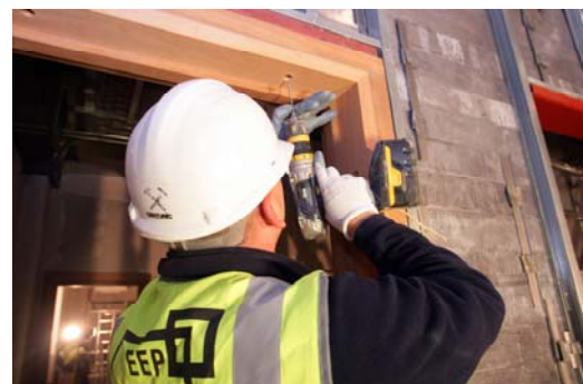
EEP offers a full installation service
