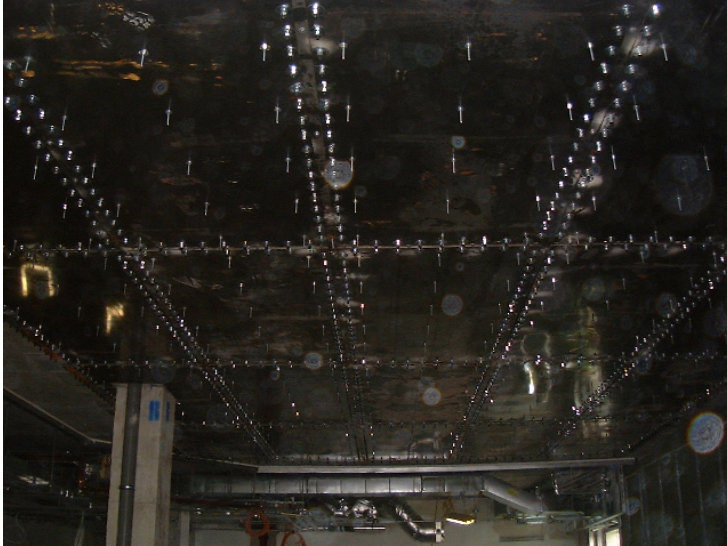
Views of magnetic field shield fixed to the ceiling slab below MRI scanners. Designed to contain the 5Guass line from the MRI extending into the room below.
