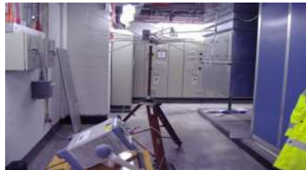
Measuring Emissions from Equipment in a Plant Room
