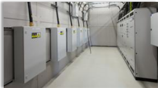
Installed Filter Array
